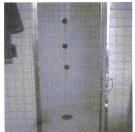
An elaborate shower features three rows of three showerheads each, plus an additional one overhead.
