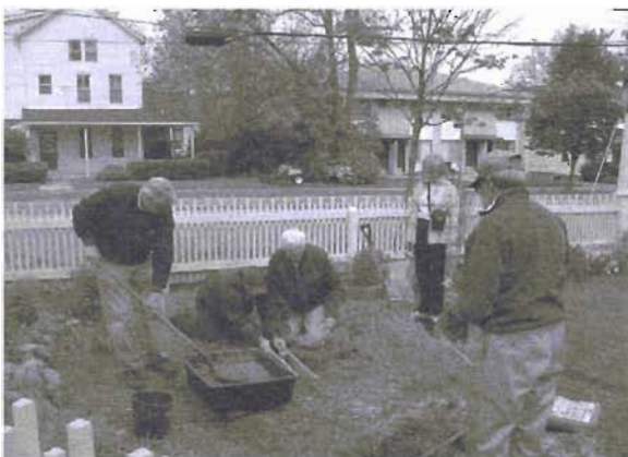
Dean Greb shovels cement into the post hole while Dick Galant and Ralph Beebe make sure the post remains level. Sue Kosky and Jay Snyder observe.
