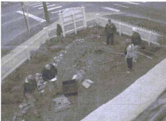
Jay Snyder and Dean Greb check directions for mixing cement for the flagpole post hole while Dick Galant, Ralph Beebe and Sue Kosky check out the site.
