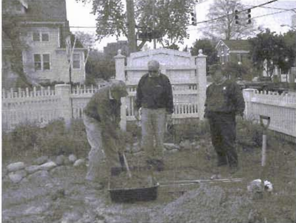
Jay Snyder mixes cement under the watchful eyes of Dean Greb and Dick Galant.
