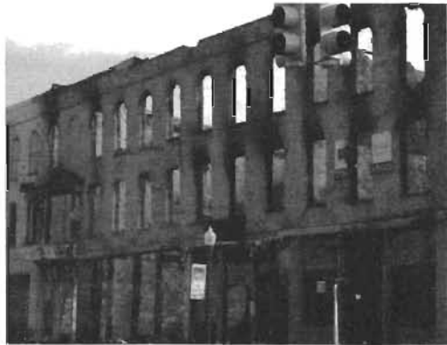
This three-story, Civil War-era building, known as the Thompson Block, sits at the eastern edge of Depot Town in Ypsilanti. The city is currently gearing up to make a decision to begin work on the project in three phases: Phase 1 will stabilize the structure; Phase 2 involves rebuilding the structure to its condition prior to a fire last fall; Phase 3 includes renovations and build-out of tenant spaces.
